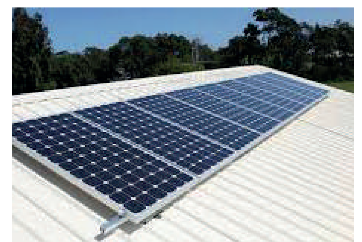
New external solar panels
